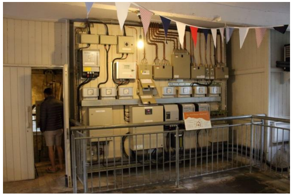
The Complex Control System for the Electricity Generation
